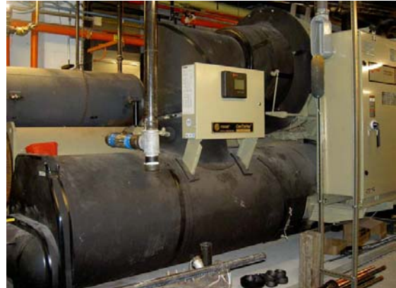
One of two 400 ton VSD-controlled electric chillers that will keep Fordham's student body cool this summer.
